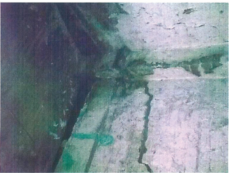
Struct. cracking from settlement in North boundary wall
