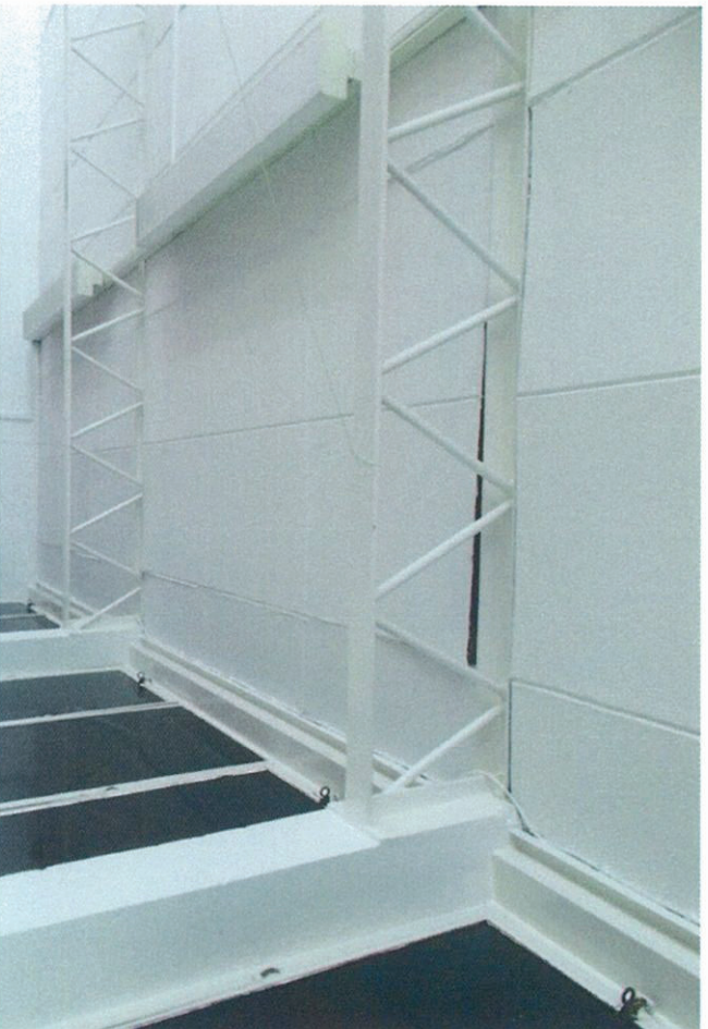
Photo 14 Failing Ceiling Boards
