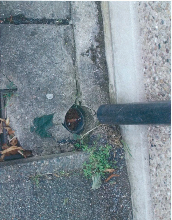
Photo 9 Example of Broken Downpipe
