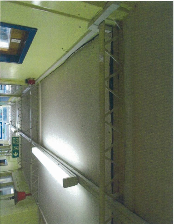
Photo 13 Failing Ceiling Boards
